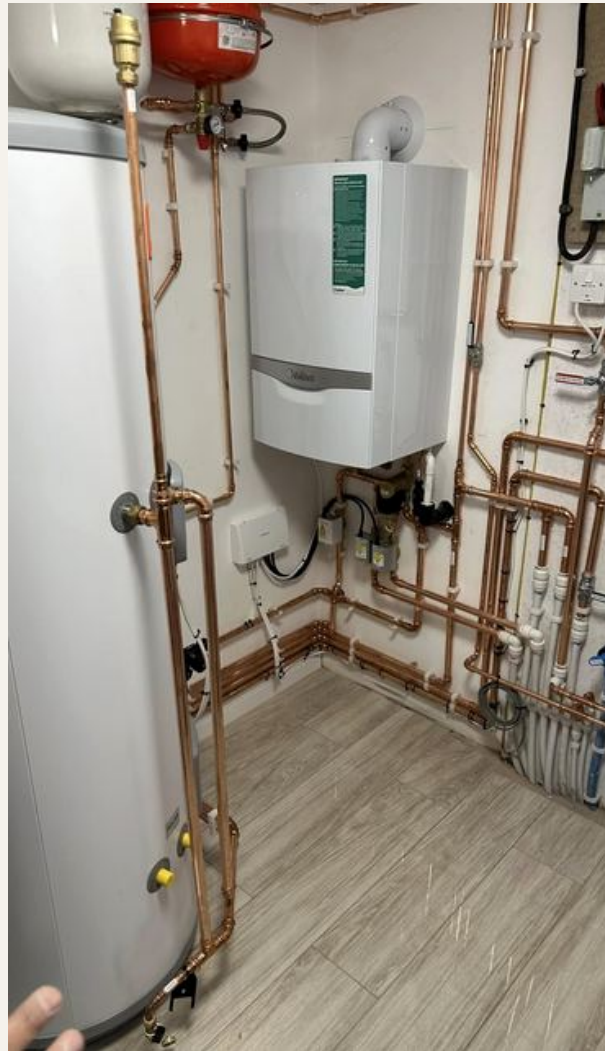
EXPOSED COPPER PIPEWORK
